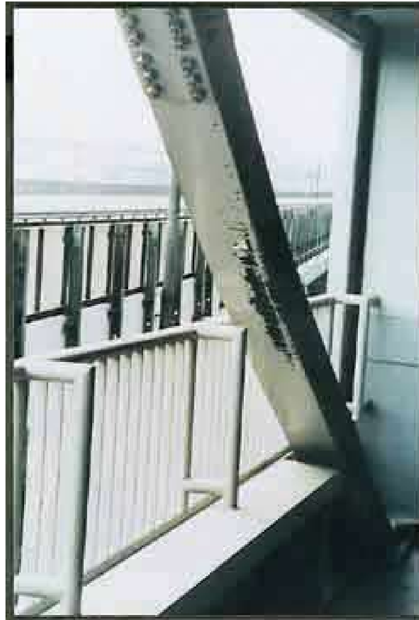
H形鋼筋違の座屈
